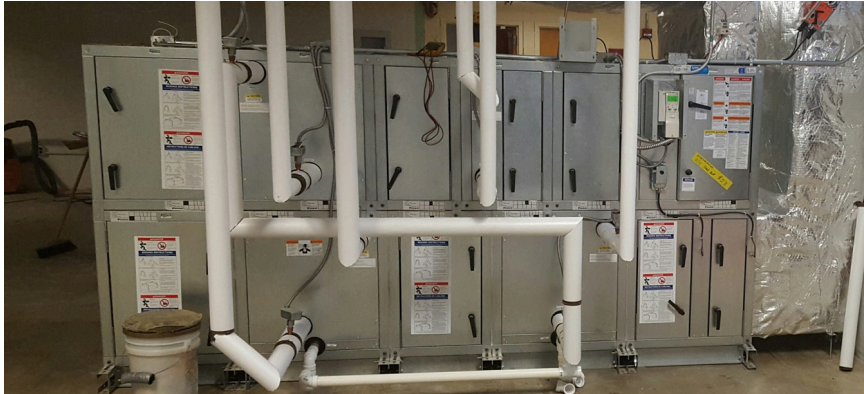
The modular TRICOIL air handlers, reassembled in the Cottage E basement mechanical room.
