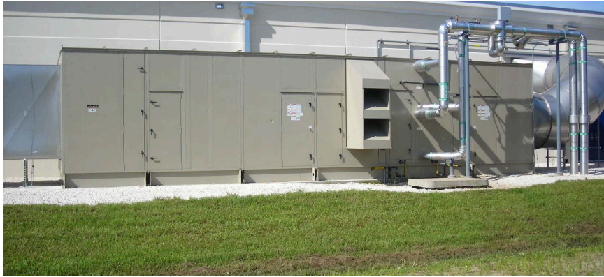
The outdoor TRICOIL air handling unit, with the insulated TRICOIL loop piping at right.
