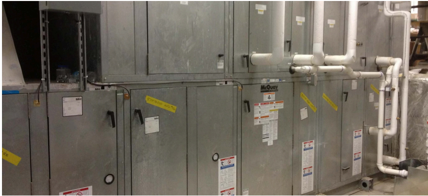
The DOAS unit installed in the building's mechanical room, with the TRICOIL loop piping at right.
