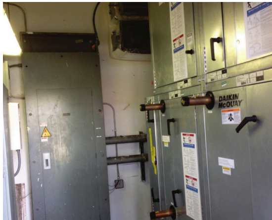
A chapter house TRICOIL air handler in its equipment room.
