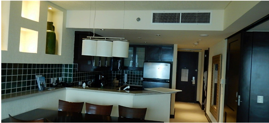
A one-bedroom villa. Its living room fan coil supplies through the grille above the kitchen; a second unit serves the bedroom.
